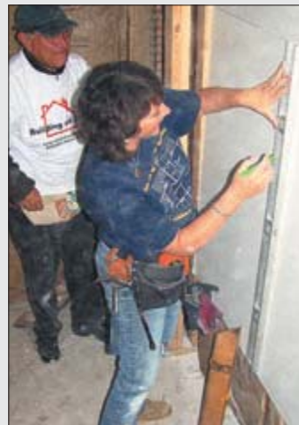
Habitat supervisor Gina Valenze hangs wallboard with volunteer Bob Silz from First UMC, Amityville.
